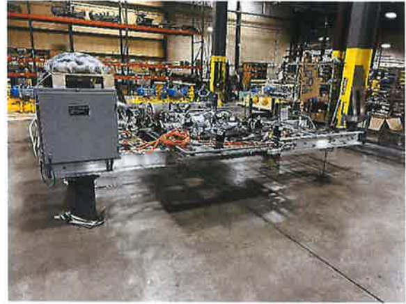
Gas Turbine Generator Fuel Control and Natural Gas manifold
